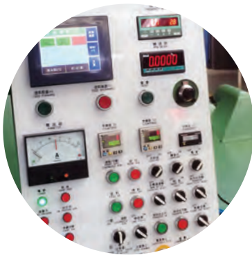
Control Panel with HMI System
